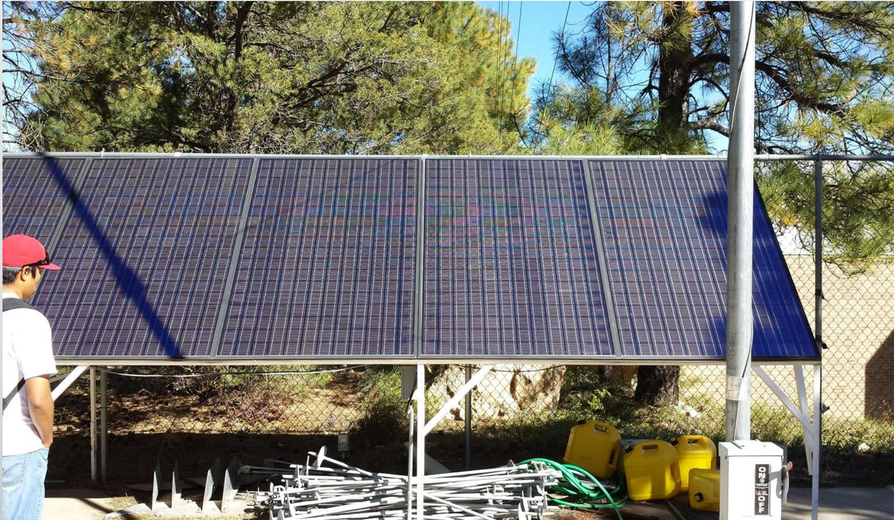
Solar Panels located up at the “Shack”
